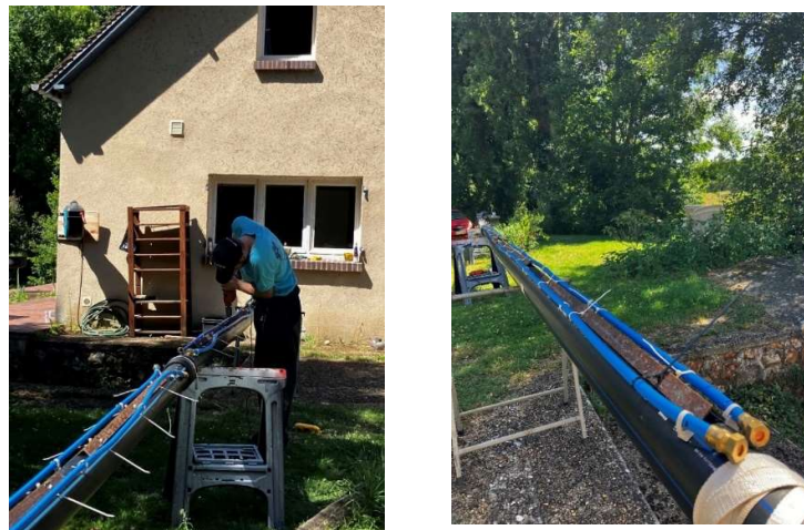
Figure 27 : Photos of the installation of the angles and bars on the SWAC tube
